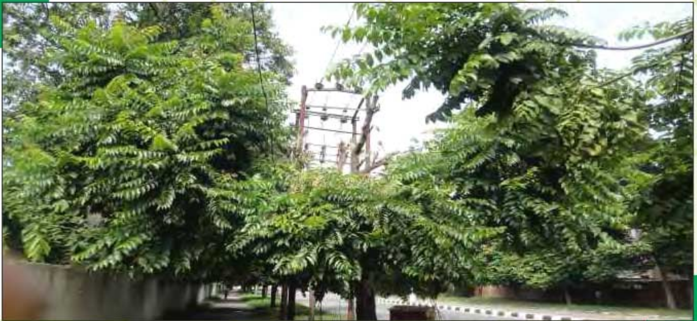
Picture 4: Conflict between tree and over head lines
